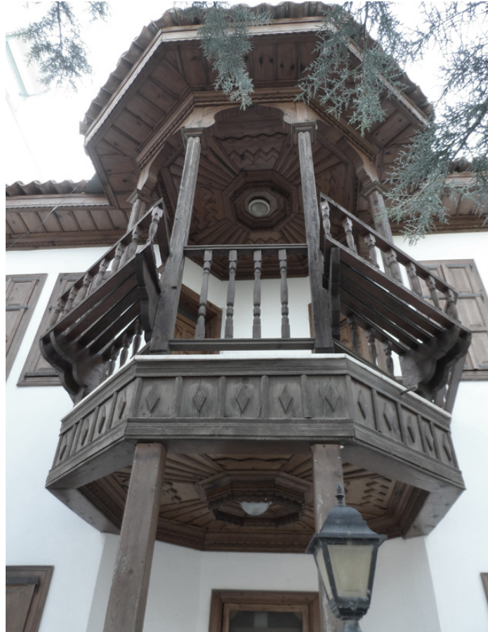
Figure 4. An imitation of sofa as balcony with too many ornamental details.
